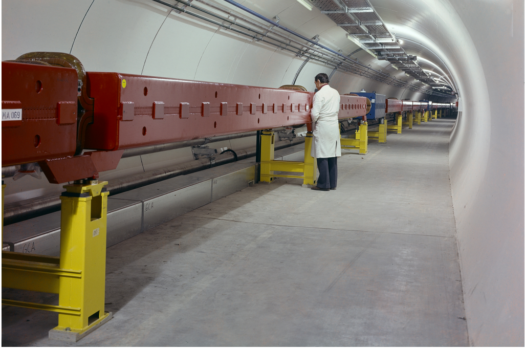
Figure 1.3.: View inside the SPS tunnel. Dipole magnets are painted red, quadrupole magnets are blue.
