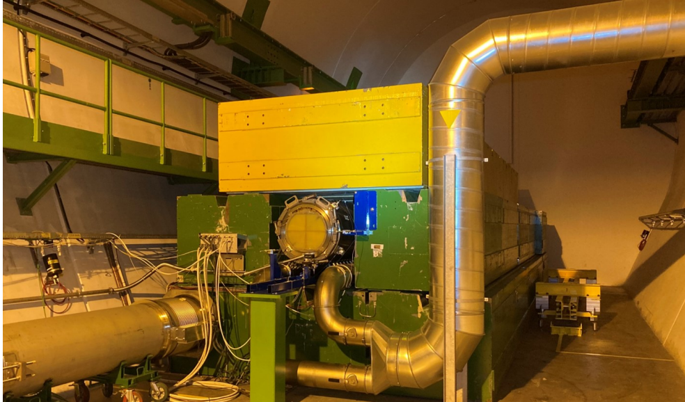
Figure 4.3: One of the beam dumps installed in its underground cavern inside the iron shielding. The circular front face visible in this image is the upstream window upon which the beam impacts first. The cooling pipes are led into the shielding area.
