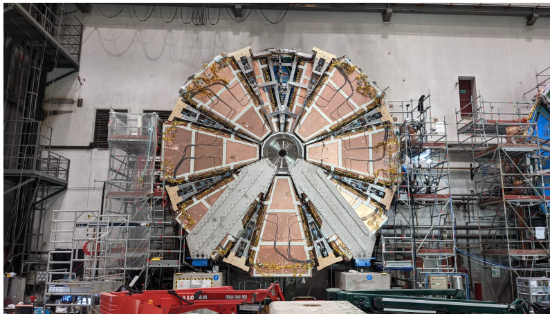
(c) A picture of one of the two NSWs. All sectors except one large sector at the top are installed, revealing two of the smaller sectors that are normally hidden under the large sectors and support bars. The NSWs are 9.3 m in diameter.
