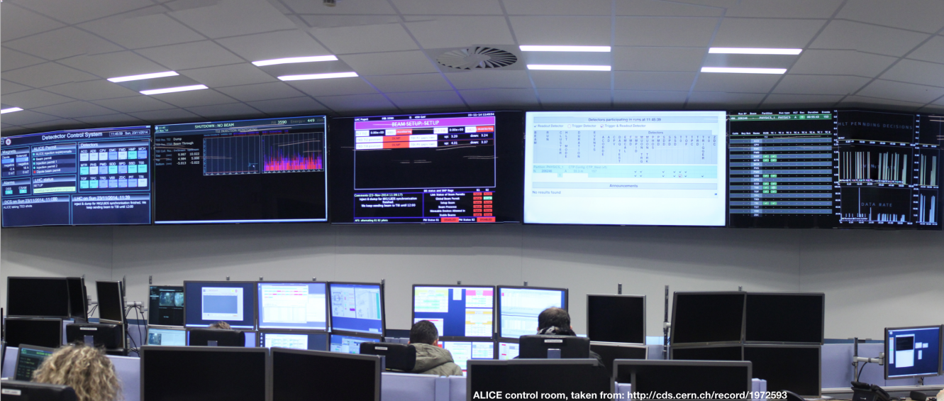
ALICE control room, taken from: http://cds.cern.ch/record/1972593
