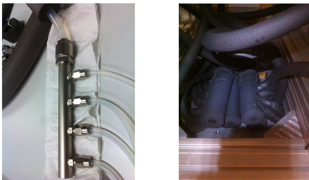
Figure 3.47: Left – Photo of the distributors of the BGV cooling system taken during the lab tests. Right – Photo of the set of insulated distributors installed in the bottom rack of the BGV setup at the LHC tunnel.
