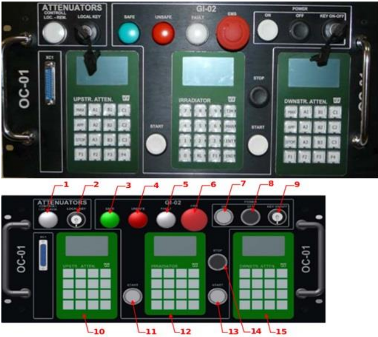
Figure 1. Front view of the OC-01 operators control. Control elements No. 3, 4, 5, 6, 7, 8, 9, 11, 12, 13 and 14 are assigned to the GI-02 gamma irradiator indication and control. Control elements No. 1, 2, 10 are 15 are assigned to the RA-01 attenuator indication and control.
