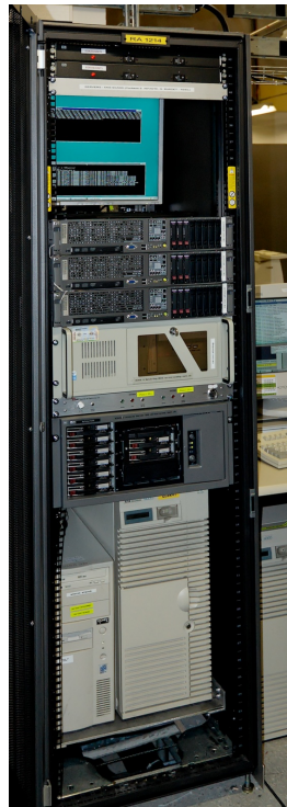
Figure 2.9: Servers of the SCADA system.
