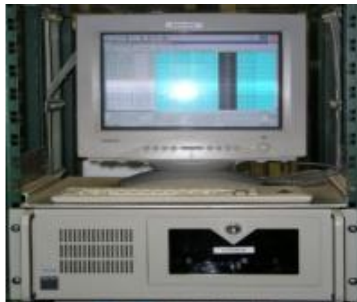
Figure 2.4: One RTU located in a surface electrical substation.
