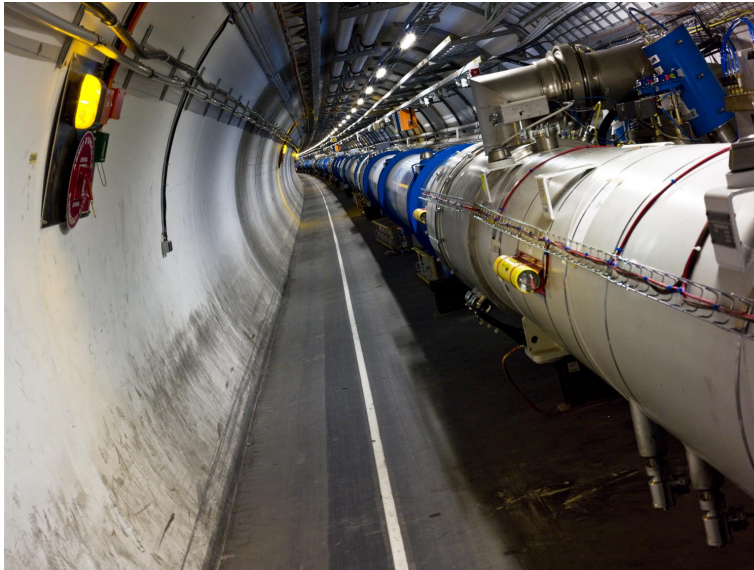
Figure 1.2. Photograph of the LHC accelerator taken in the tunnel. Copyright CERN PhotoLab, Maximilien Brice.
